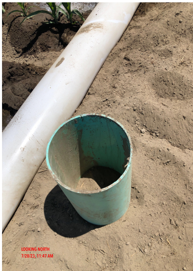
Photo 12 Piping along southern edge of Subject Property
